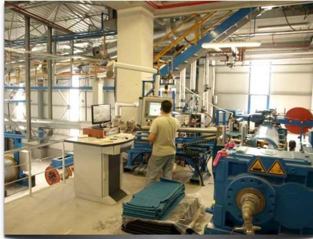
CV line extruder room
